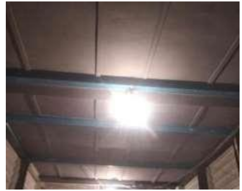
CEILING BATON FOR LIGHTS
